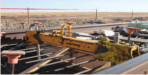
Iron Horse Engineering casting frame supporting rail and tie plate assemblies for concrete casting
