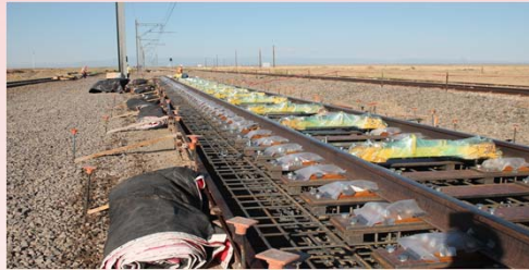
Photos showing top rebar mat and coverage of critical components prior to casting of concrete.
